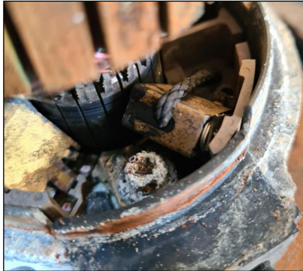
Figure 19: Example of signs of corrosion within the motor enclosure.
