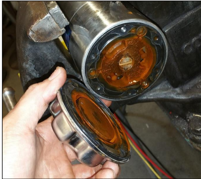
Figure 17: Example of signs of rust within the motor enclosure which is also a sign of unwanted water entering the motor enclosure.
