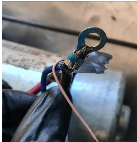
Figure 18: Example of poor wiring quality (no solder, poor crimping, not insulated, etc.)
