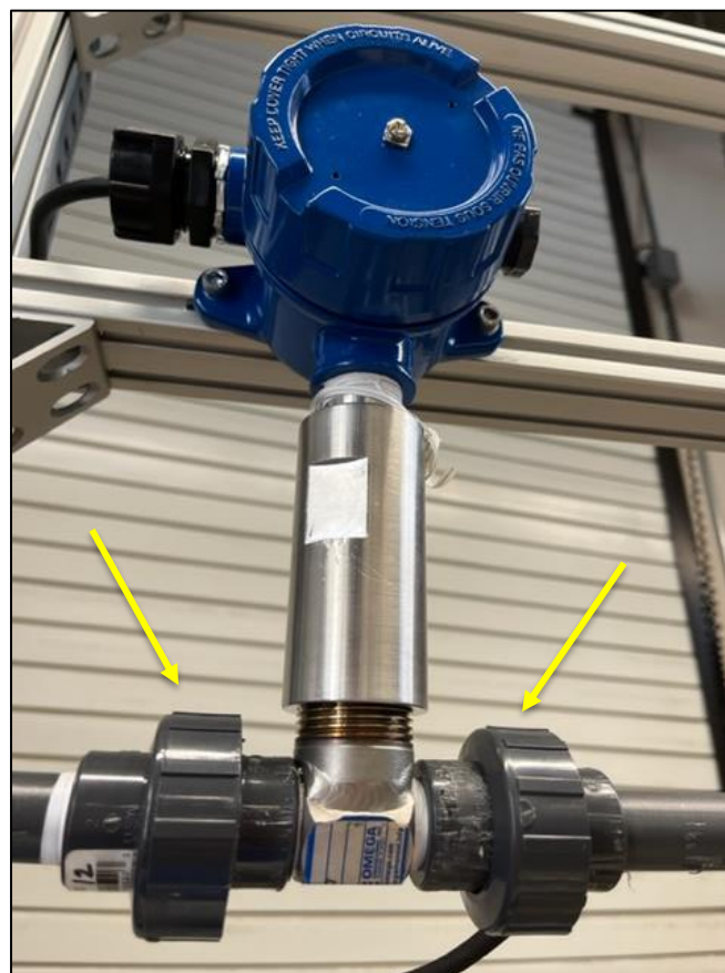
Figure 5. Flow meter and PVC adapters on either side for ease of removing/ re-installing it to the test bench PVC network.
